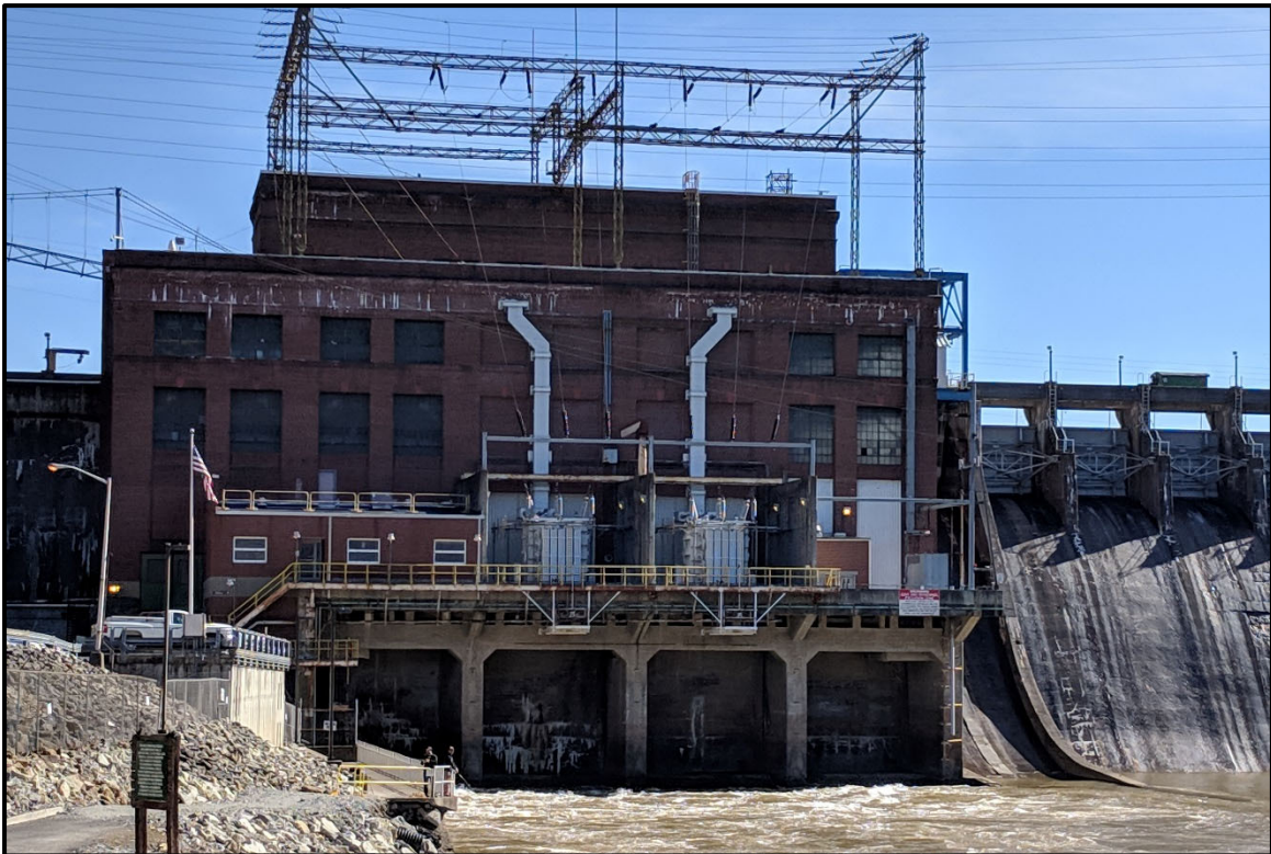
Figure 5. View of Powerhouse at Lake Lynn Hydroelectric Project.
