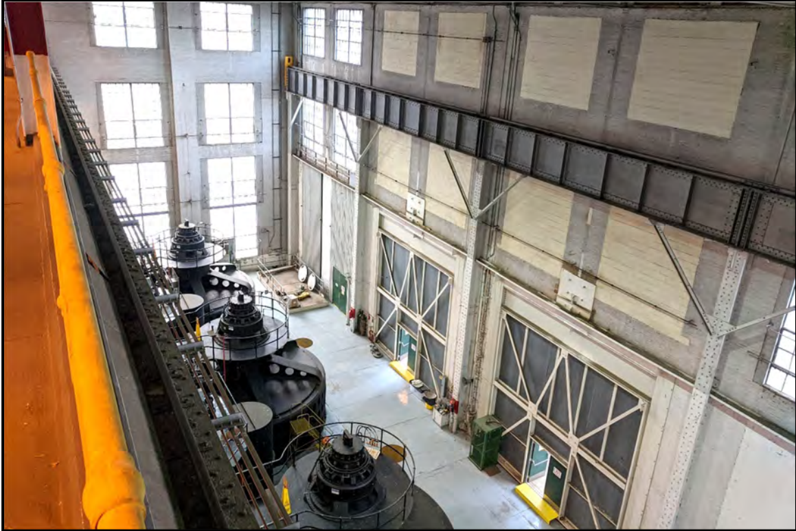
Figure 6. View of Interior of Powerhouse at Lake Lynn Hydroelectric Project.
